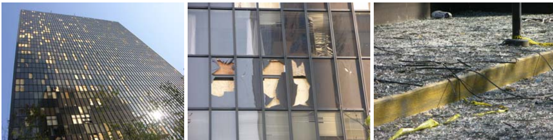
Figure 11 – High-rise building on Poydras Street (near the Hyatt) – the debris at base was both broken glass and gravel
