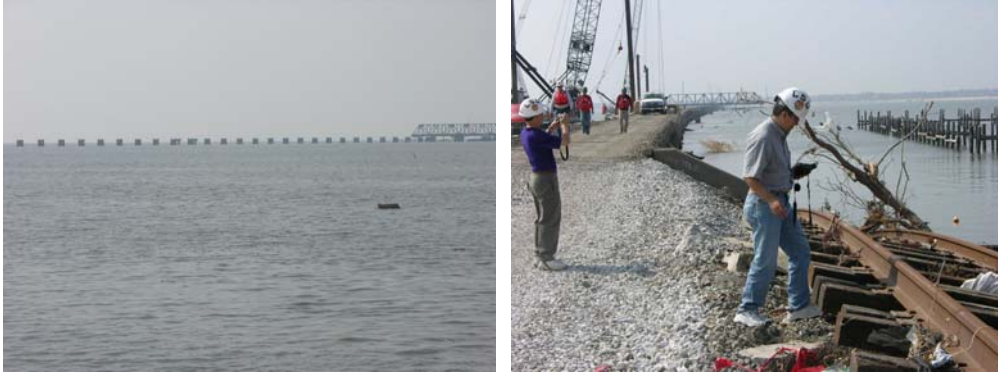
Figure 3 - Rail bridge across Bay St. Louis (reconstruction in progress), from the East End
