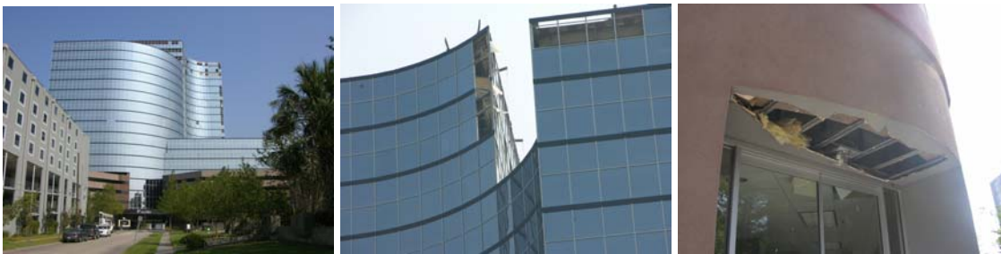
Figure 6 - Cladding damage to the Galleria building at the north end of New Orleans
