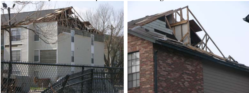
Figure 5 - Gable end roof failures in neighborhoods north of New Orleans
