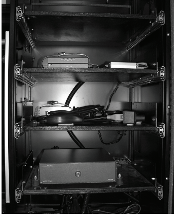
Figure 2: DieselNet equipment in a bus locker
