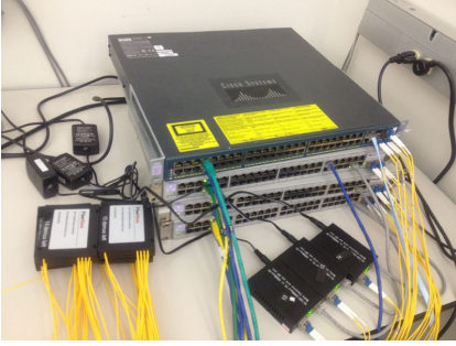
Figure 11: Quartz with 4 switches, connected by WDMs
